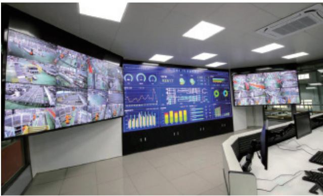
Intelligent monitoring center
